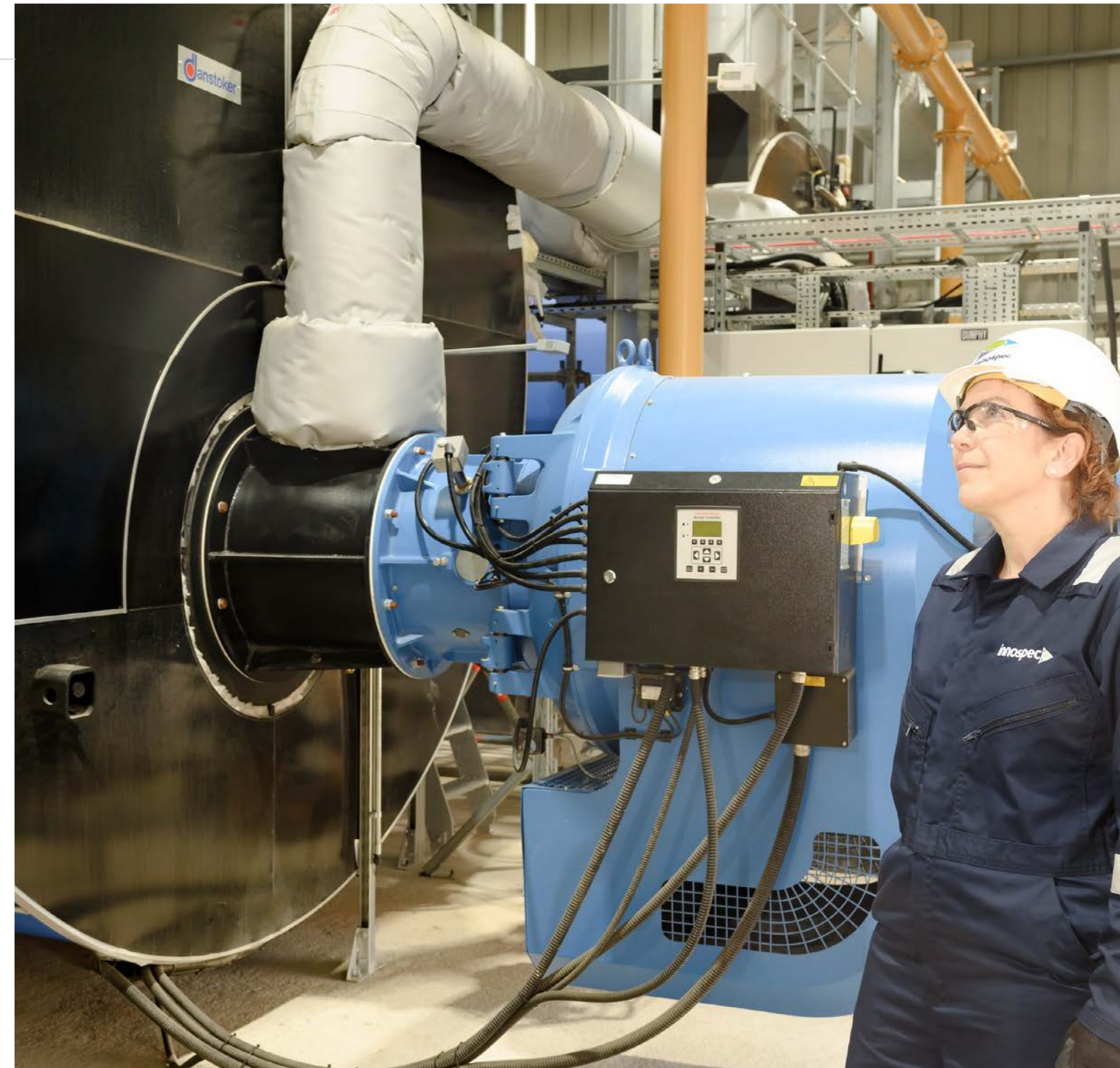
Our Ellesmere Port, UK, site completed the first phase of the installation of a new Energy Centre including a combined heat and power (CHP) plant. Janet Newton our site Engineer, project managed the design and build of the plant.
